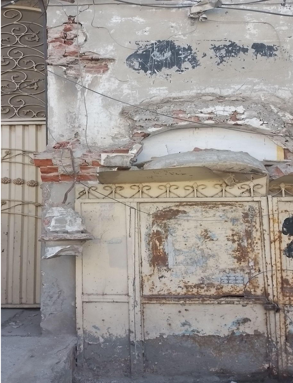
Demolished minarets at an Ahmadiyya site of worship in Baghbanpura, Gujranwala
